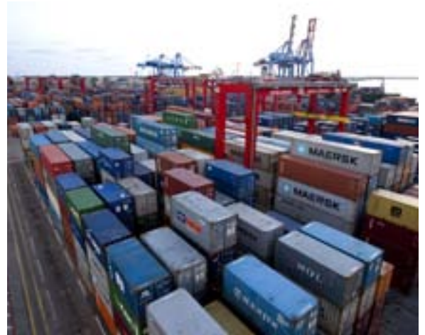
Four new Konecranes RTG cranes are being assembled at the Abidjan container terminal.
